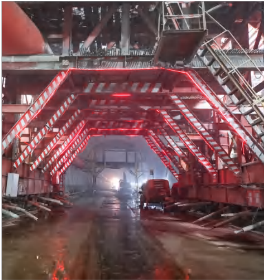
Steel Formwork Tunnel Trolley
